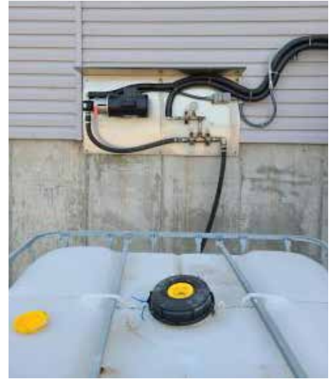
PDS 1 - An oil system on a fertilizer building
