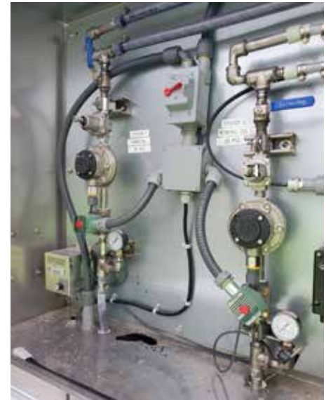
PDS-C1S - This system has 2 application points inside this box
